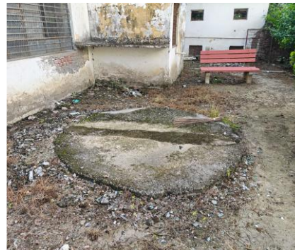
Wainwater Harvesting Pit
