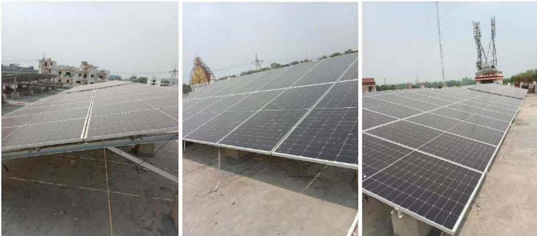
Solar Panels installed in different campuses of Gurukula Kangri (Deemed to be University), Haridwar
